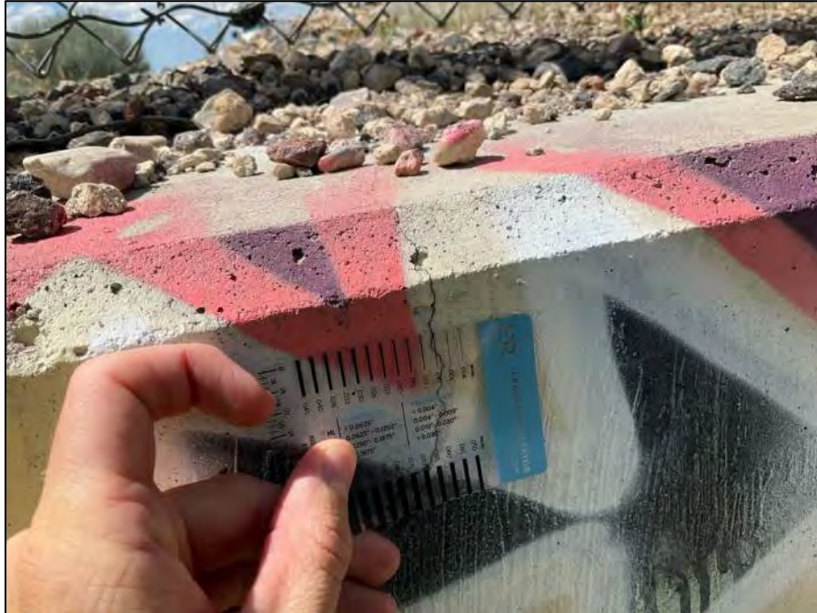
Figure 2 – Narrow Vertical Cracking in North Abutment
