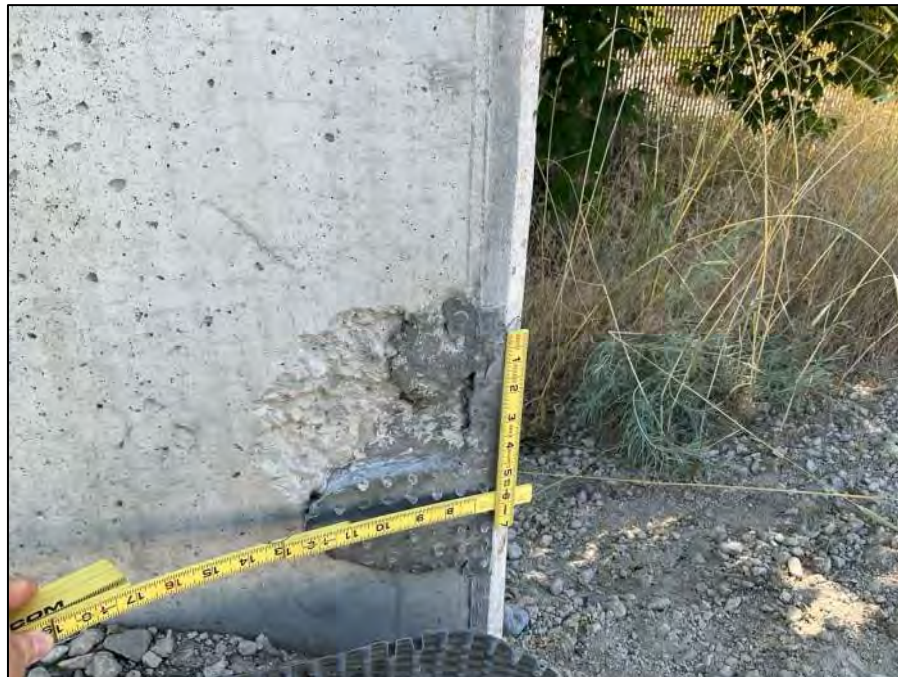
Figure 3 – Shallow Spall in Northwest Wingwall
